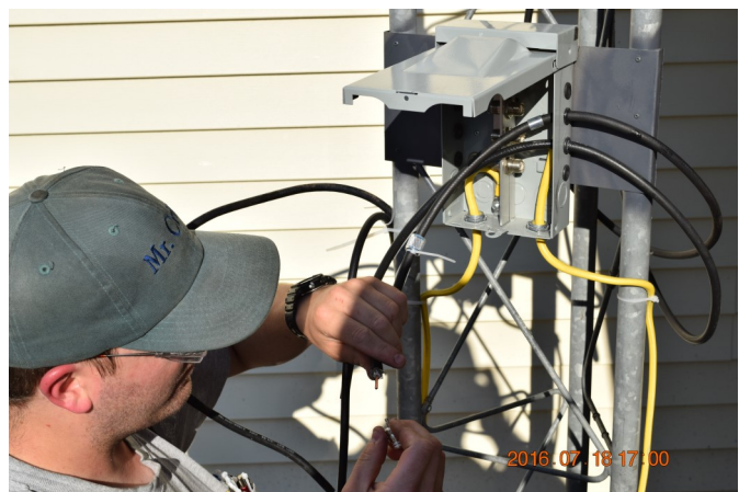
Joe had already pulled the cables from his shack. Peter finished work by terminating the cables.
